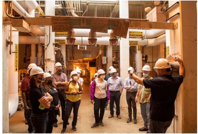
MWRD Commissioners Kimberly Du Buclet and Eira L. Corral Sepúlveda and staff tour a new heat exchanger system at a digester complex at the Calumet Water Reclamation Plant. The system will consume less energy and generate savings through the MWRD's sustainable generation of biogas to heat facilities.
