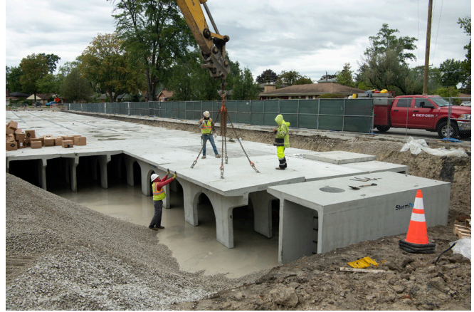
The MWRD is investing in innovative stormwater management solutions, such as the Marvin Parkway Flood Control Project in Park Ridge. Here, the MWRD is partnering with Park Ridge to construct an underground storage facility that helps mitigate flooding and retain water.
