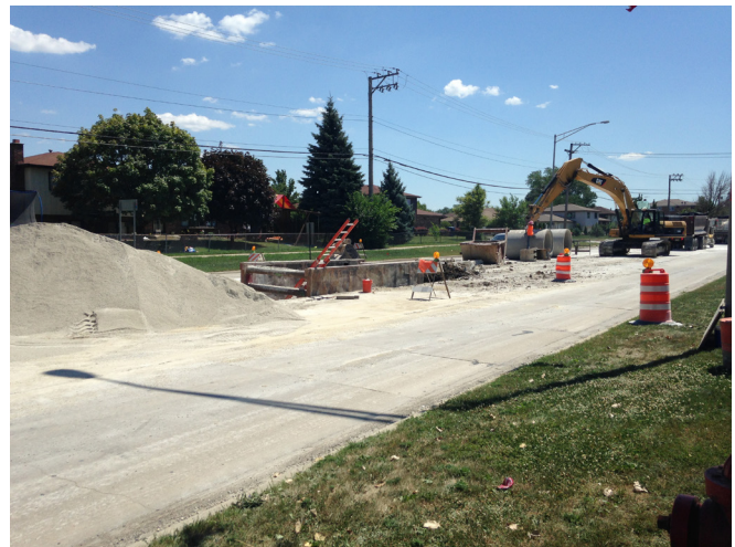
A new storm sewer is installed below Roberts Road to provide flood relief to commercial and residential structures in the villages of Justice and Bridgeview as part of the MWRD's Stormwater Partnership Program.
