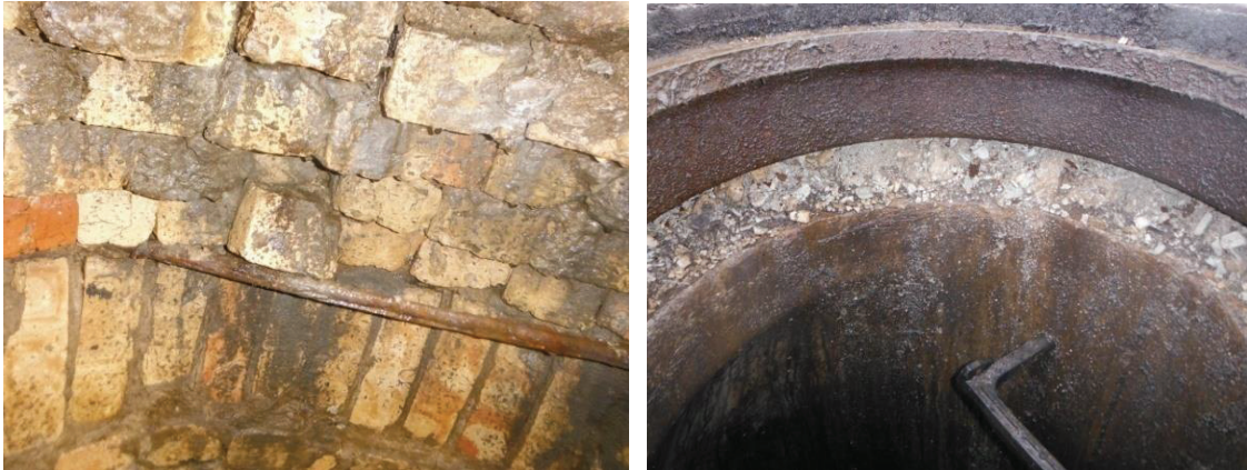
Figure 8.7. High-Priority Manhole Defects – Left: Deteriorating Brickwork; Right: Deteriorated Adjustment Ring
