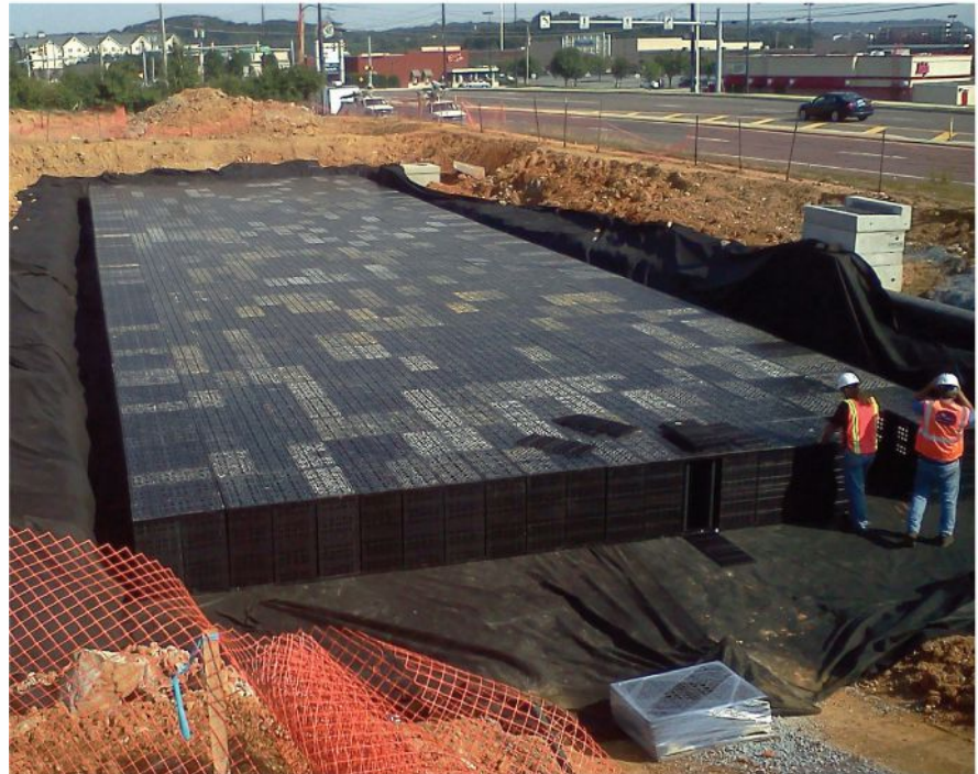
The system provides nearly 20,000 cu ft of storm water storage.
