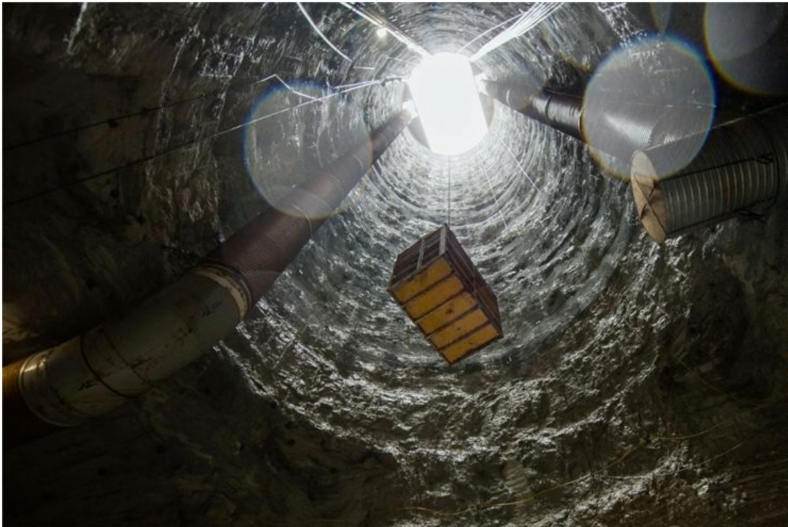
Workers are raised and lowered into the Des Plaines Tunnel via a cage-like container hoisted by crane.
