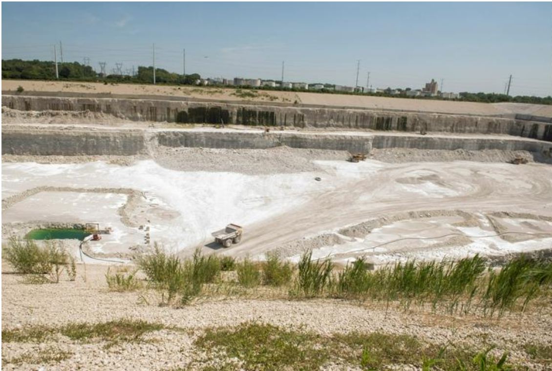
McCook Reservoir Stage II is being mined to create more capacity for the MWRD. Approximately 55 million tons of rock have been removed, as more than 60 percent of the mining work still awaits.
