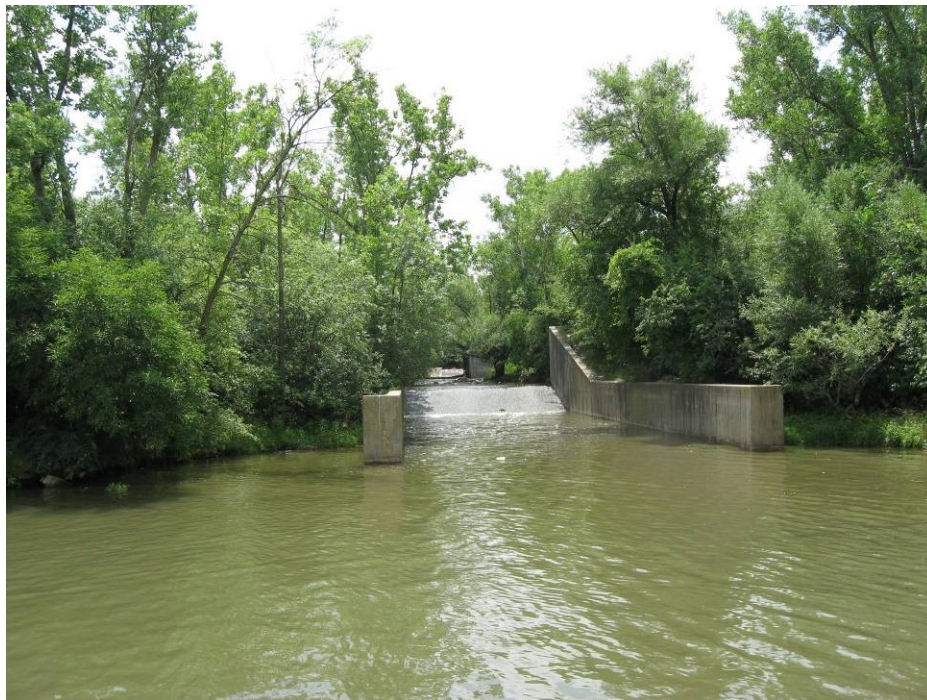
Figure 2-16: Tributary Access Blocked by a Concrete Structure at the Mouth of Tinley Creek on the Cal-Sag Channel (photo taken 2008).
