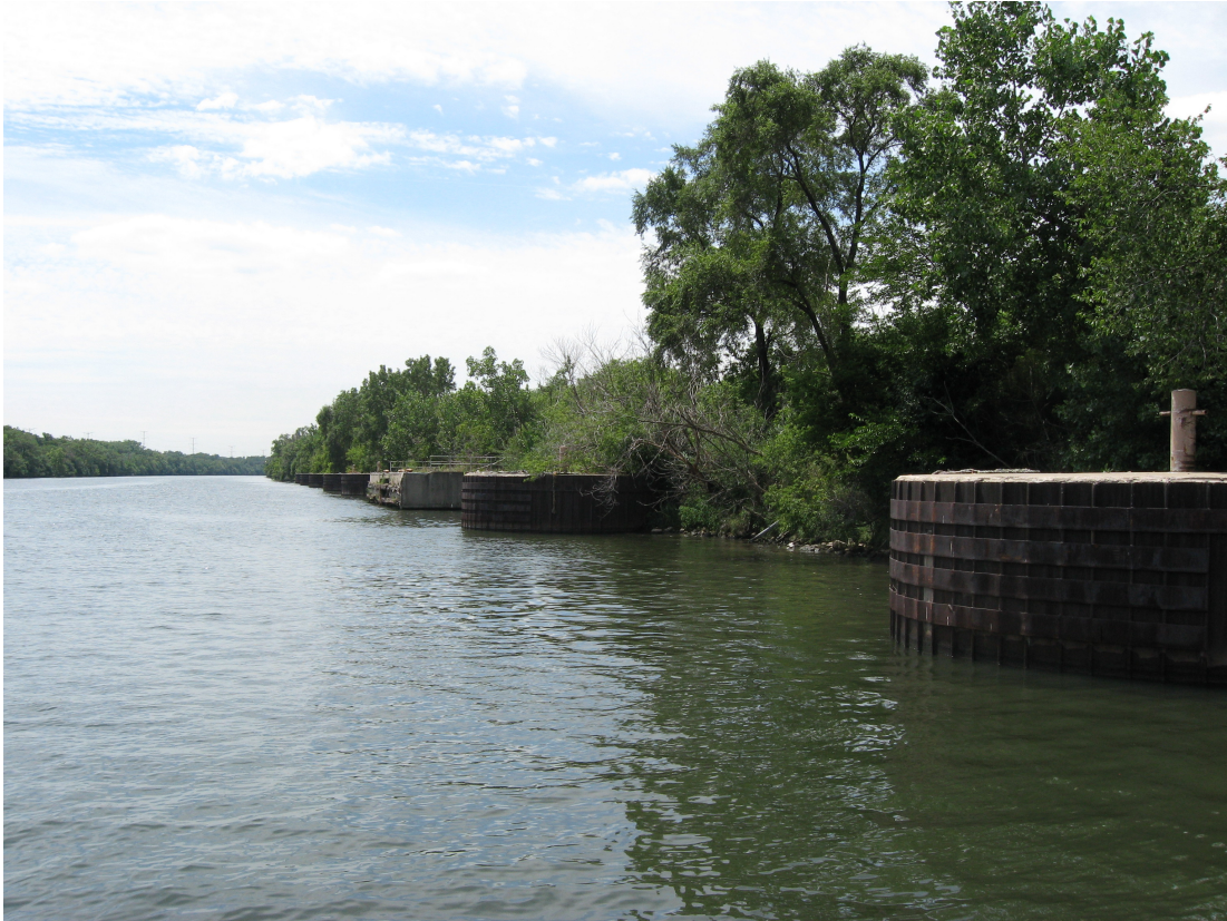
Figure 2-2: Examples of Dolphin Structures on the Chicago Sanitary and Ship Canal near AWQM 41.
