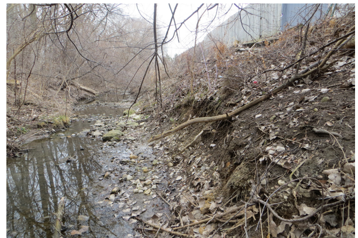
Crestwood Drainage Ditch will be repaired and stabilized.
