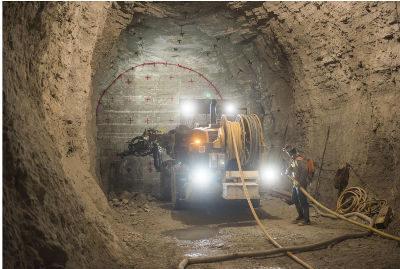
Excavation for the Des Plaines Dewatering Tunnel on May 9, 2017, which would eventually connect to the McCook Reservoir, a major component of the MWRD's Tunnel and Reservoir Plan (TARP).
