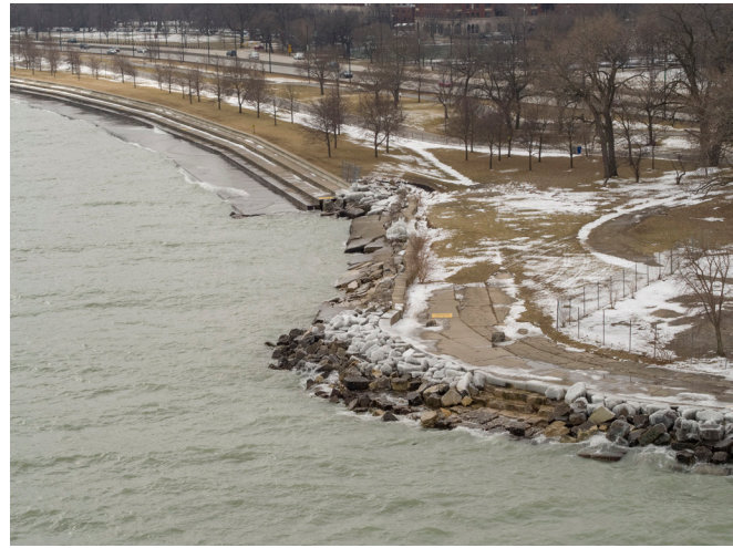
The MWRD will fund much needed lakefront restoration caused by high lake levels and damaging waves that occurred during major storms in January 2020.
