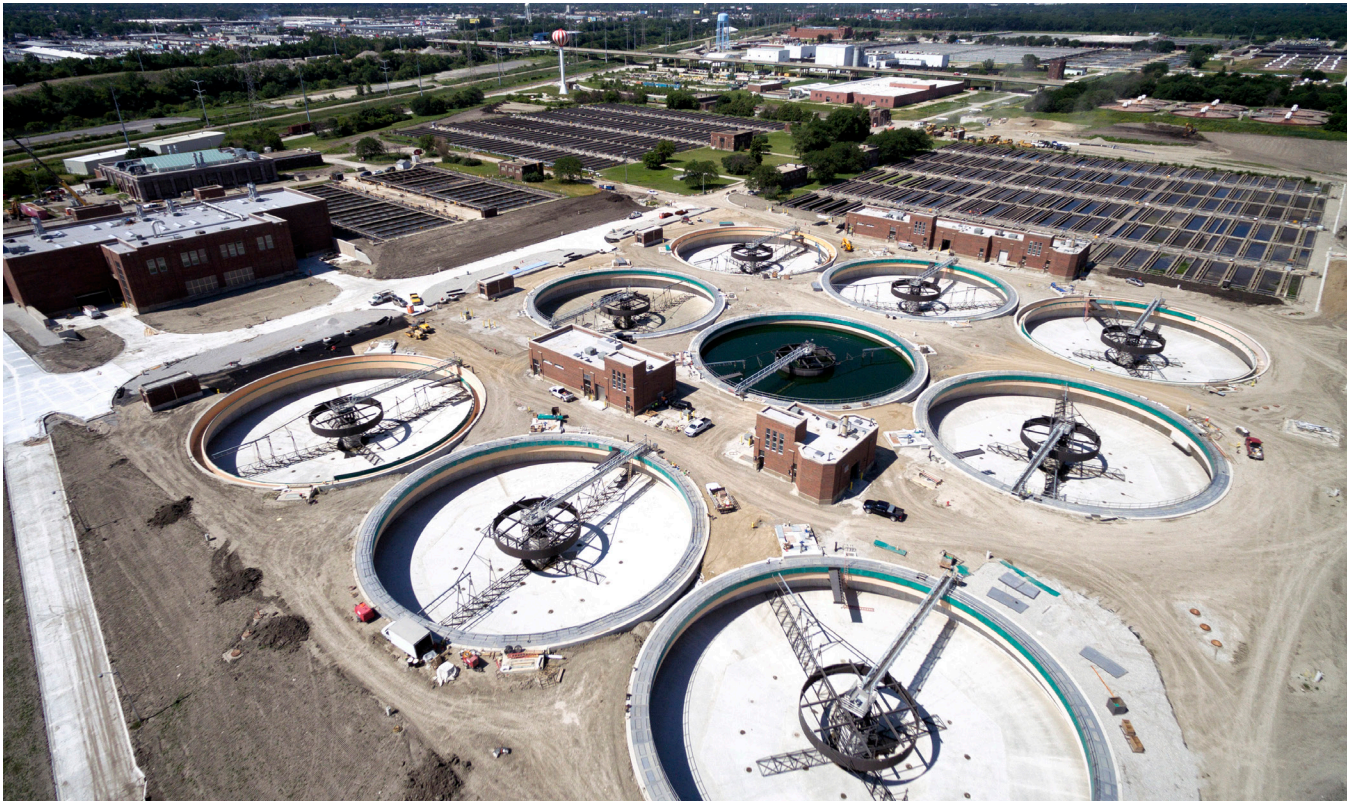
New primary settling tanks at the MWRD's Stickney Water Reclamation Plant help the MWRD lower its carbon footprint by trapping methane emissions and reproducing energy that can be returned to the plant.
