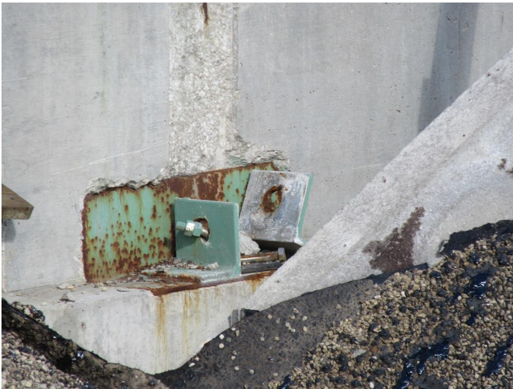
b) Damaged connection at failed single tee over GBT Room
