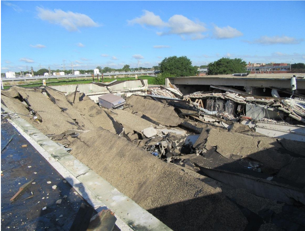
Figure 1. Overall view of collapsed structure at GBT Room looking east
