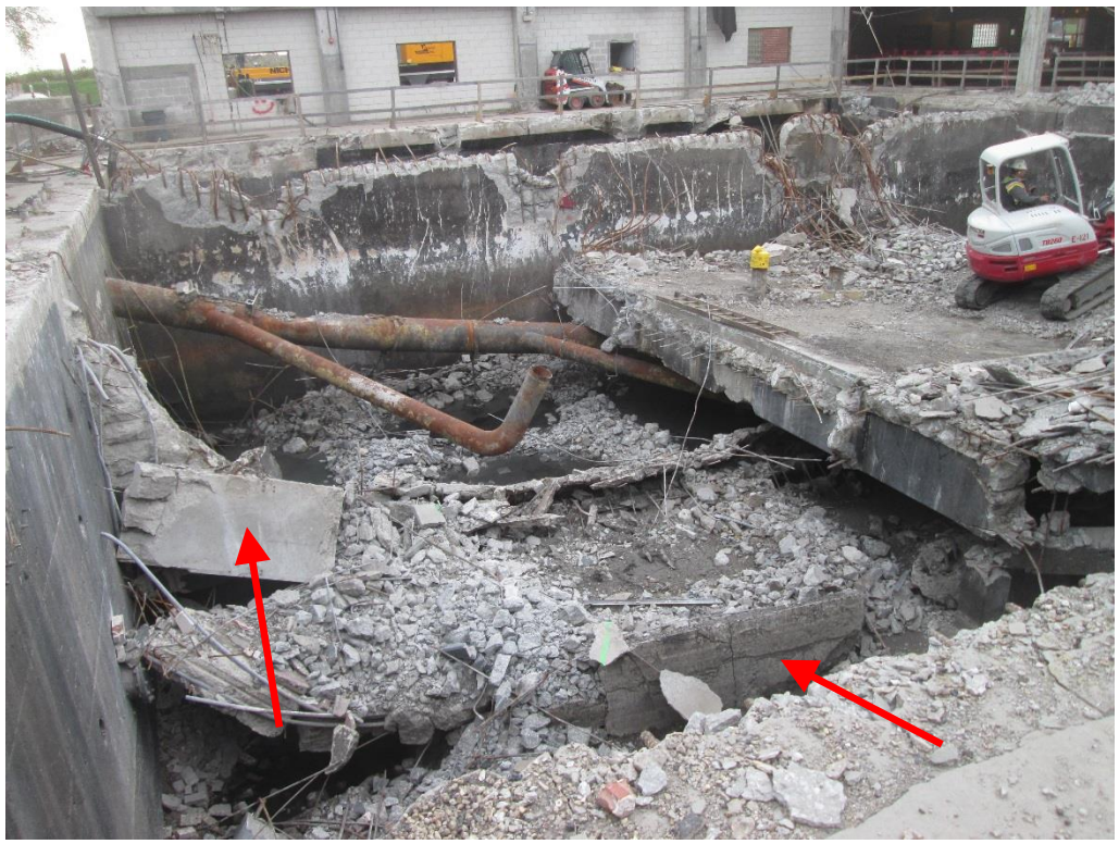
Figure 32. Top of wall separating west tank from center tank with no epoxy grouted dowels present
