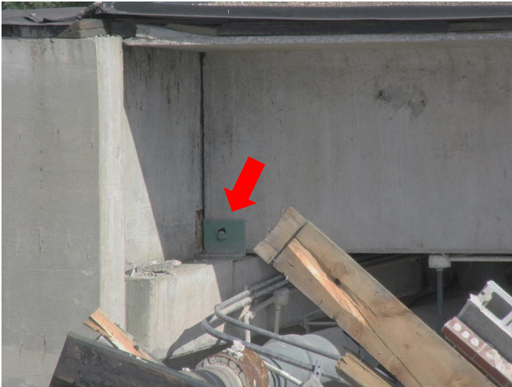
a) Undamaged connection for single tee roof beam over Sludge Screen/Polymer Rooms
