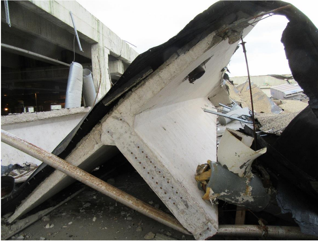
Figure 12. East end of single tee roof beam fallen from bearing on east wall
