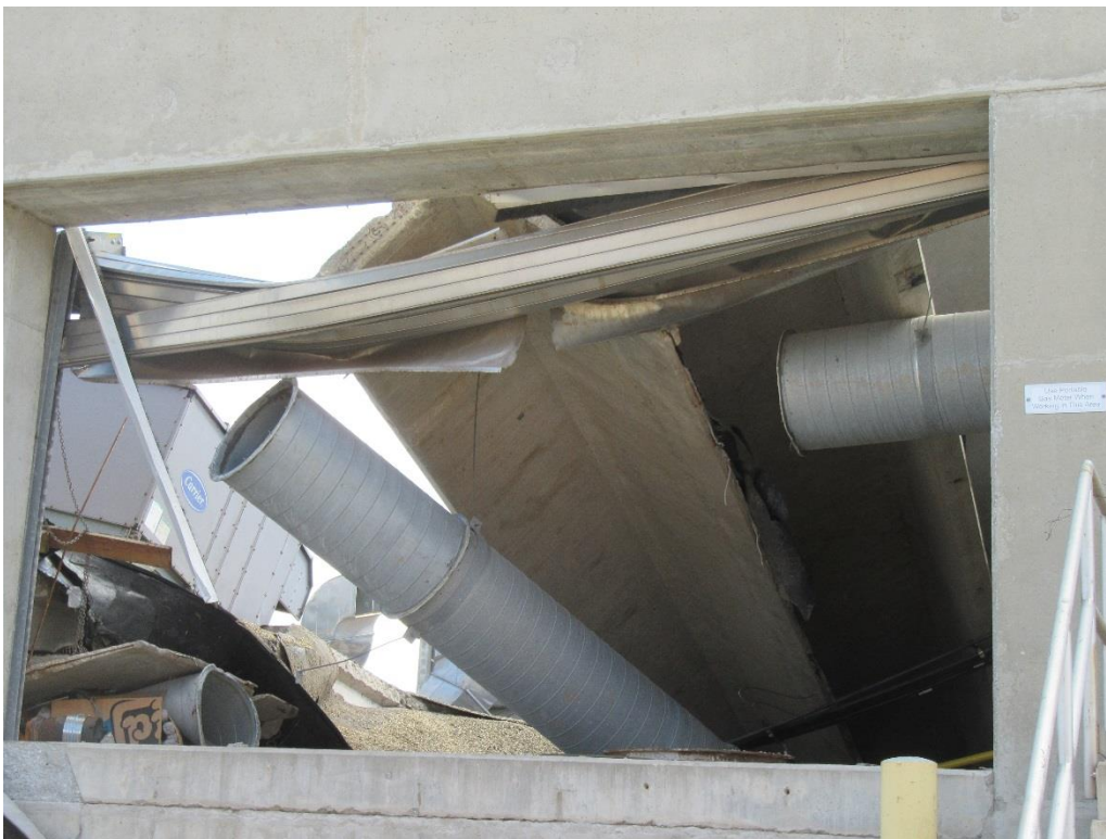
Figure 13. West end of collapsed single tee Roof Beam 5 and 6 supported on rolling overhead door
