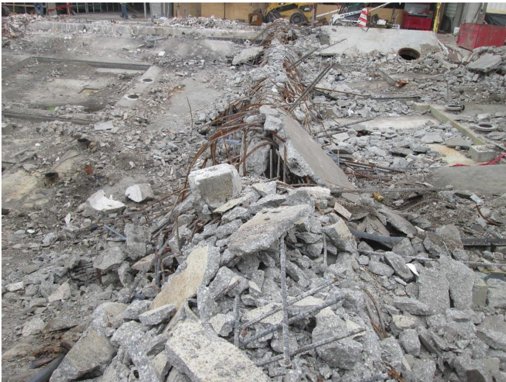
Figure 21. Damaged floor slab over interior wall between east and center tanks
