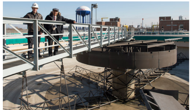
(L-R) MWRD Principal Civil Engineer Paul O'Brien and MWRD Commissioner Frank Avila survey a new primary settling tank.
