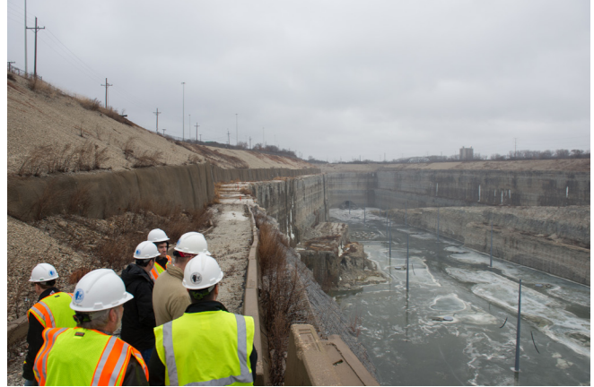
MWRD engineers stand at the southwest corner of Stage I of the McCook Reservoir as it begins to take on water for the first time on January 11, 2018.
