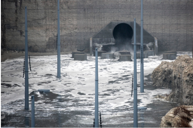
McCook Reservoir Stage I started to take on water at approximately 9:30 a.m. from the Mainstream Tunnel System just minutes after the gates were opened from the tunnel on January 11.
