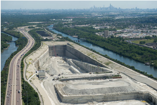
McCook Reservoir will become a destination for stormwater and wastewater to prevent it from polluting local waterways, but to make that happen miners and haulers had to remove 1.8 million cubic yards of overburden from the 30.6 acre excavation site.
