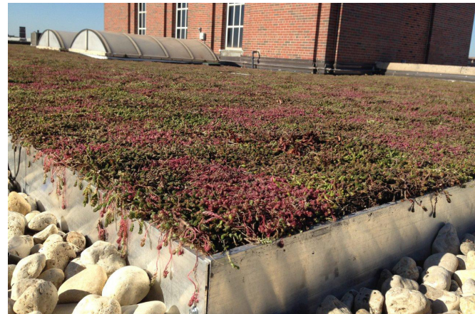
The green roof at the MWRD's Racine Avenue Pumping Station, a building that houses equipment that pumps wastewater to the Stickney Water Reclamation Plant. The structure's total building roof area is 33,000 sq. ft., and approx. 4,500 sq. ft. is structurally-rated to handle the additional vegetative roof loading.
