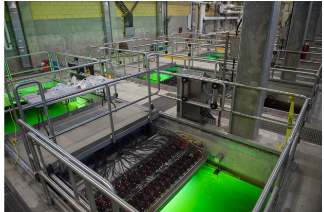
New ultraviolet technology implemented at O’Brien Water Reclamation Plant will provide another layer of protection by disinfecting treated water that flows through channels that emit a green glow as a result of the system being optimized for light in the UV spectrum and not normal visible white light.
