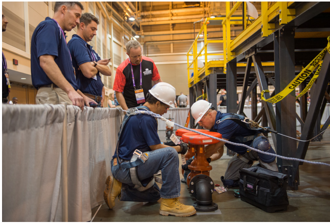
L-R: Ed Staudacher and Matt Jurjovec cheer on John Conry and Josh Filler as they repair a check valve in the safety competition during the Operations Challenge event held at the Water Environment Federation Technical Exhibition and Conference in New Orleans last month.
