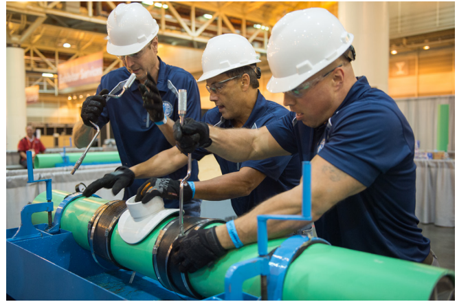
L-R: John Malinowski, John Conry and Josh Filler install a new section of pipe in the collections event during the Operations Challenge held at the Water Environment Federation Technical Exhibition and Conference.
