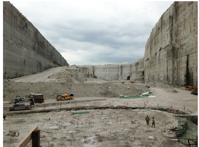
The first section of the McCook Reservoir, holding 3.5 billion gallons, is nearing completion in 2017. The reservoir is part of the Metropolitan Water Reclamation District of Greater Chicago's Tunnel and Reservoir Plan (TARP) that captures and stores combined stormwater and sewage that would otherwise overflow from sewers into waterways in rainy weather or local basements.
