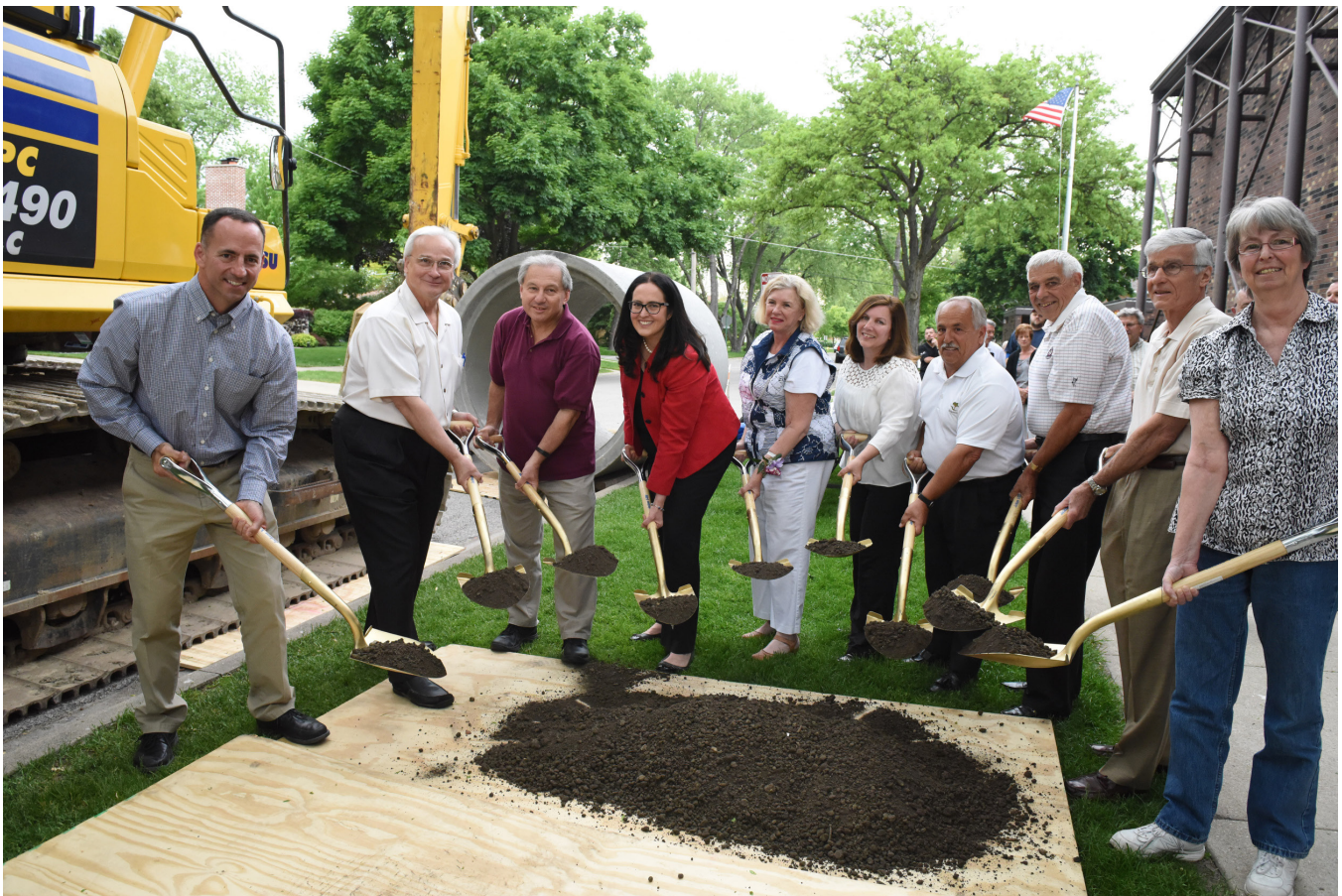
Metropolitan Water Reclamation District of Greater Chicago President Mariyana Spyropoulos joined officials with the village of Niles, the Forest Preserves of Cook County and the Illinois Environmental Protection Agency to break ground on a 11,200 feet of new storm sewer that will minimize surface water flood damages in Niles and improve water quality in the North Branch of the Chicago River.
