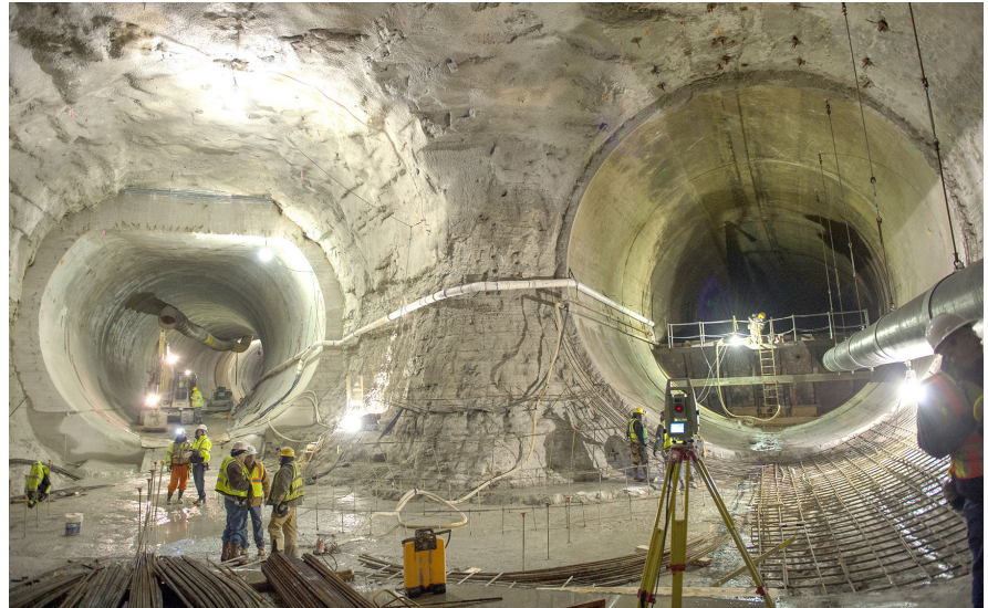
Construction workers complete the confluence of the McCook Reservoir Connecting Tunnel (left) and the Mainstream Tunnel (right) as part of the MWRD's Tunnel and Reservoir Plan. New funds provided by Congress' Omnibus Appropriations bill for 2016 will allow the MWRD to complete the McCook Reservoir's first stage by 2017.
