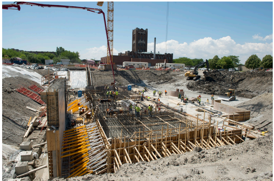
Crews begin forming the foundation to one of two new facilities that will house part of the MWRD's new ultraviolet disinfection facility at O'Brien Water Reclamation Plant in Skokie. The new facility will improve the quality of treated water entering the North Shore Channel.
