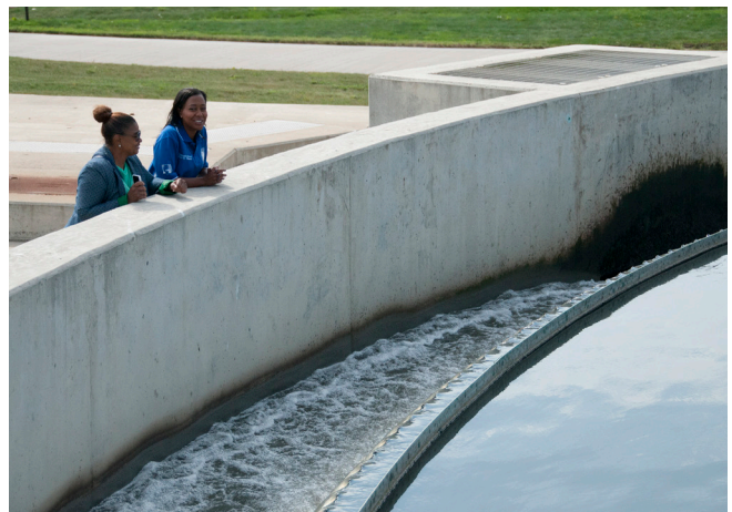
In the photo: Aide to Commissioner Kari Steele, Nikkida Hart, and Commissioner Steele survey a final settling tank, one of the last steps of the wastewater treatment process, at the Calumet Water Reclamation Plant in Chicago on Sept. 20.
