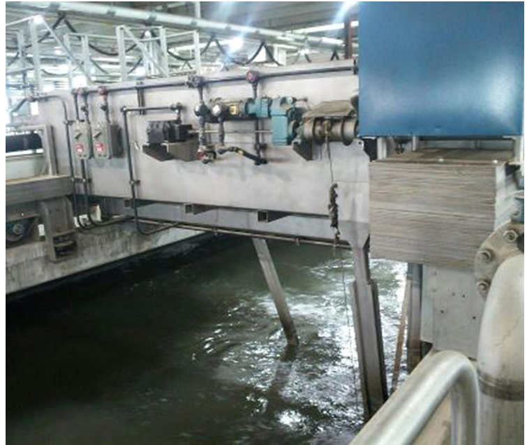
Pictured is a new traveling grit bridge at the Calumet WRP. This bridge moves automatically back and forth along the grit chambers helping to remove inorganic particles that could harm equipment or interfere with downstream processes.
