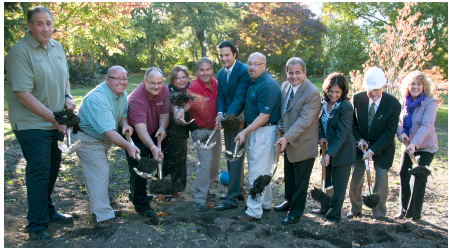
MWRD Commissioner Michael Alvarez (6th from left) joined City of Berwyn and Berwyn Park District officials for the Proksa Park water drainage improvement project groundbreaking on Oct. 2.
