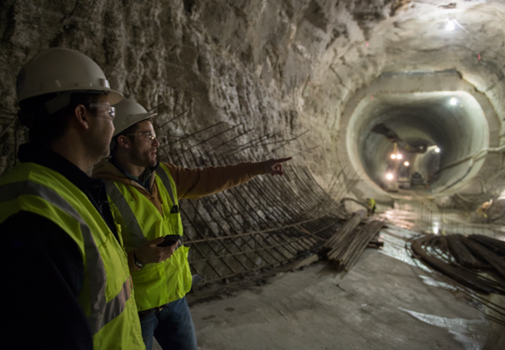
The MWRD's vision extends hundreds of feet below ground through the Tunnel and Reservoir Plan, working to reduce flooding, improve water quality in Chicago area waterways and protect Lake Michigan from pollution.
