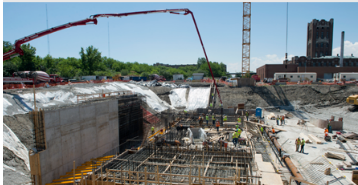
In its work to reclaim water, the MWRD is constantly evolving to meet new challenges through innovation and infrastructure upgrades that allow the MWRD to raise its water quality standards and meet stringent permits.
