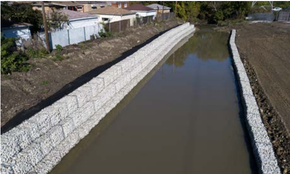
Channel improvements , which clear and widen streams to improve water flow and prevent erosion.
