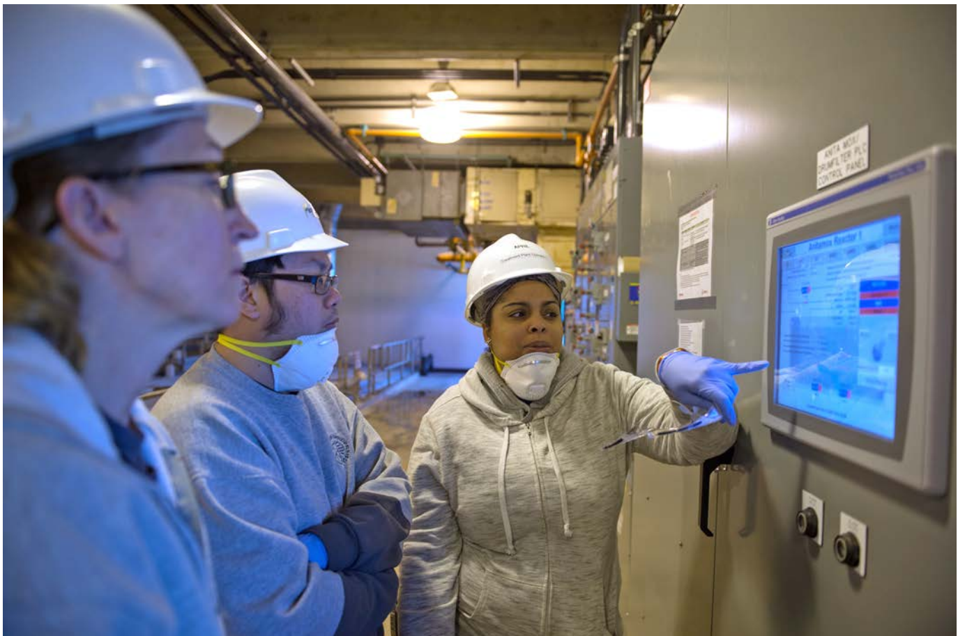
Treatment plant operators at the Egan Water Reclamation Plant discuss operations to remove nutrients from wastewater using the most efficient, economical ways possible that also reduce the District's energy and carbon use.
