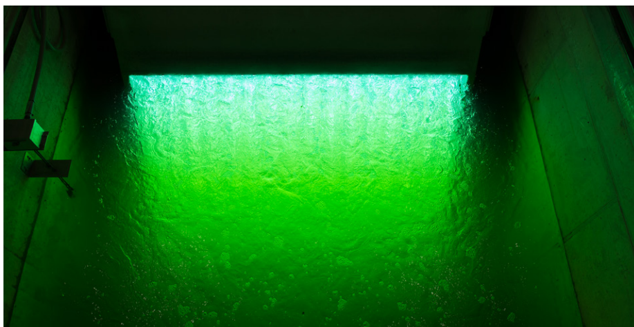
Powerful UV light neutralizes microbes in the water before it is released from the O'Brien WRP. Although UV the light itself is invisible, the 896 bulbs in the disinfection facility emit green light in the visible spectrum.
