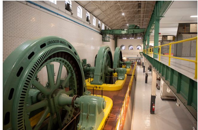
The MWRD's Lockport Powerhouse is expected to undergo $10 million in upgrades in 2020, thanks to the strong finances of the MWRD that were made possible by a responsible investment policy that will now consider sustainability factors. An example of sustainability, the Powerhouse generates approximately 40 million kilowatt hours of electrical energy annually, generating $1.2 million in revenue for the MWRD.
