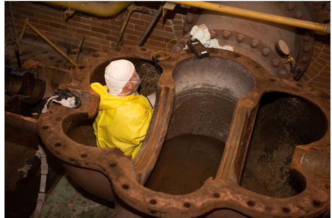
MWRD pipefitters like Vernon Hart maintain and enter pipes to ensure water is flowing properly and there are no service disruptions.
