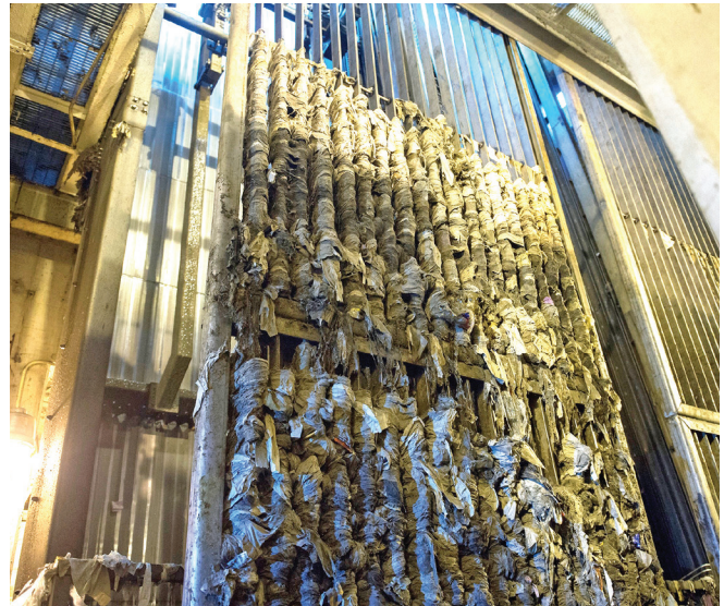
Screens are used to filter out debris as it reaches the MWRD water reclamation plants, but wipes, paper towels, tissues and other products can accumulate and stick to equipment. With more disinfecting wipes being used, the MWRD urges the public to only flush toilet paper.
