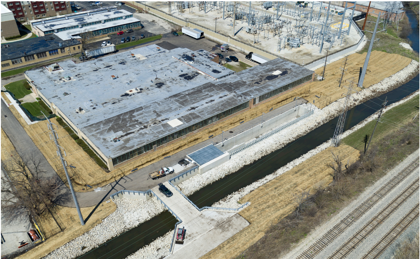
The first phase of work on the Addison Creek Reservoir and Addison Creek Channel improvement projects included the stabilization of the creek alongside the reservoir in Bellwood with a control structure, inlet structure, spillway and pumping station. When excess stormwater overwhelms the channel, it can feed into the reservoir.
