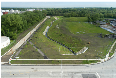
Flow from the new stormwater park and pond is controlled by three drop structures and conveyed through a culvert under 135th Street. The MWRD anticipates additional work south of the street to begin in late 2024, making way for the new park anchored around a naturalized stormwater storage pond. This pond will provide native habitats for wildlife and a place to fish and gather surrounded by other potential opportunities for recreation and economic development.
