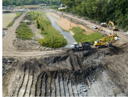
Construction on the Robbins Heritage Park and Midlothian Creek Restoration Project begins with the creation of a diversion channel. The project will significantly increase the drainage capacity in Robbins.
