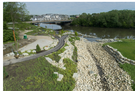
Work on the diversion channel nears completion in spring 2024, connecting flow to the Cal-Sag Channel with stone armoring along the channel waterline, a trail, waterfront access and scenic backdrop. The MWRD is transforming a generally abandoned industrial area and expanding livability with numerous enhancements. The project increases stormwater capacity, mitigates flooding, improves water quality and adds 38 acres of public greenspace with accessibility to parks, natural areas and waterways in Robbins.
