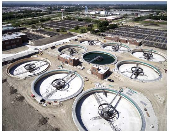
The District is constructing new primary settling tanks and aerated grit tanks, support facilities, service tunnels, and conduits at the Stickney Water Reclamation Plant. This will replace tanks, produce renewable energy, increase and improve grit removal, protect downstream piping and equipment, increase water recycling and reduce odors.
