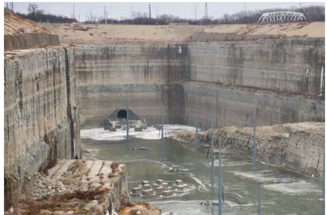
Stage 1 of the McCook Reservoir began taking water for the first time during an unusually warm January 11, 2018.
