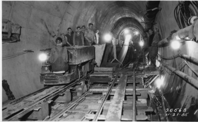
Workers pause for a photo during construction of a portion of the Southwest Intercepting Sewer on November 21, 1935.
