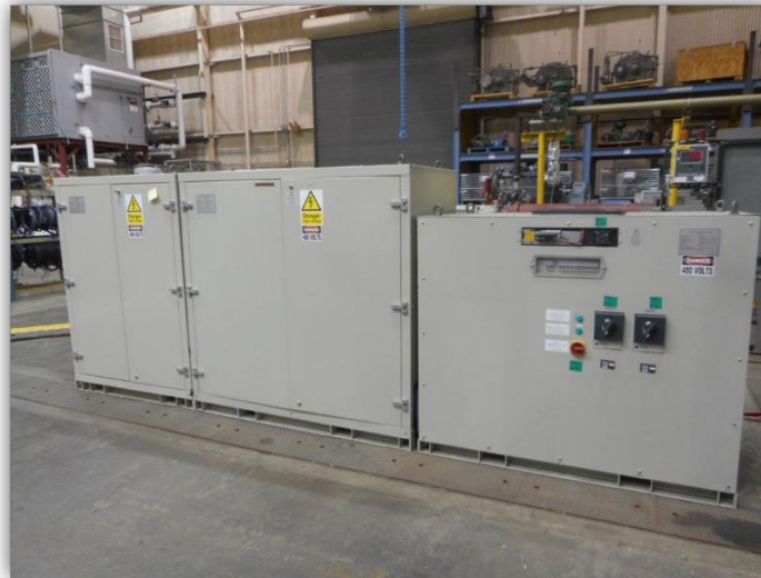
1MW VFD and power panel assembly
