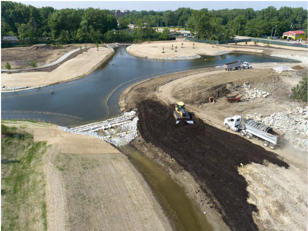
Construction progresses at the Robbins Heritage Park and Midlothian Creek Restoration Project site in June. The project will help address overbank flooding through a new stormwater park and pond, along with improvements to Midlothian Creek and an overflow channel that connects to the Cal-Sag Channel.
