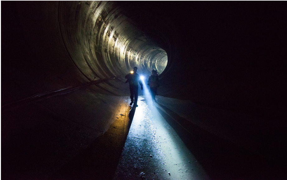
The 36.7-mile Calumet TARP tunnel system captures combined sewer overflows and carries water to Thornton Reservoir.
