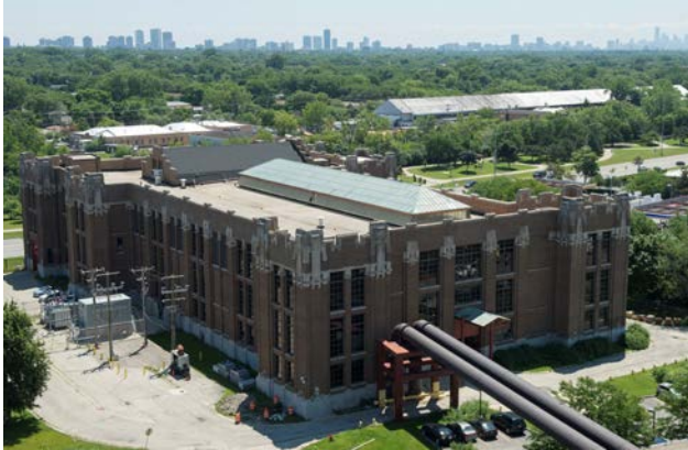
In 2020, the District will begin a $10 million rehabilitation of the steel spandrel beams in the pump and blower house at the O'Brien WRP.
