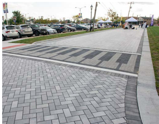
Permeable pavers on North Street, between Oak Park Avenue and 173rd Street in Tinley Park will provide 69,000 gallons of stormwater storage on site.
