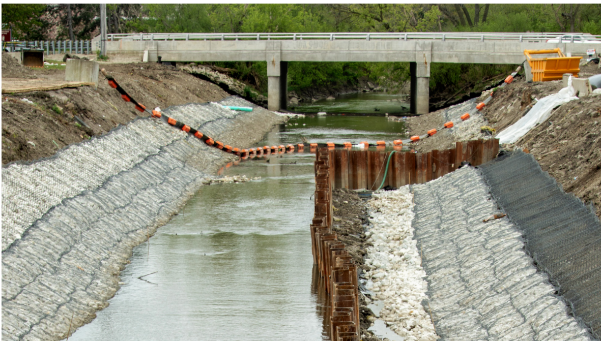
Addison Creek Reservoir and channel improvements will reduce flooding to over 2,200 structures in six communities along the creek.
