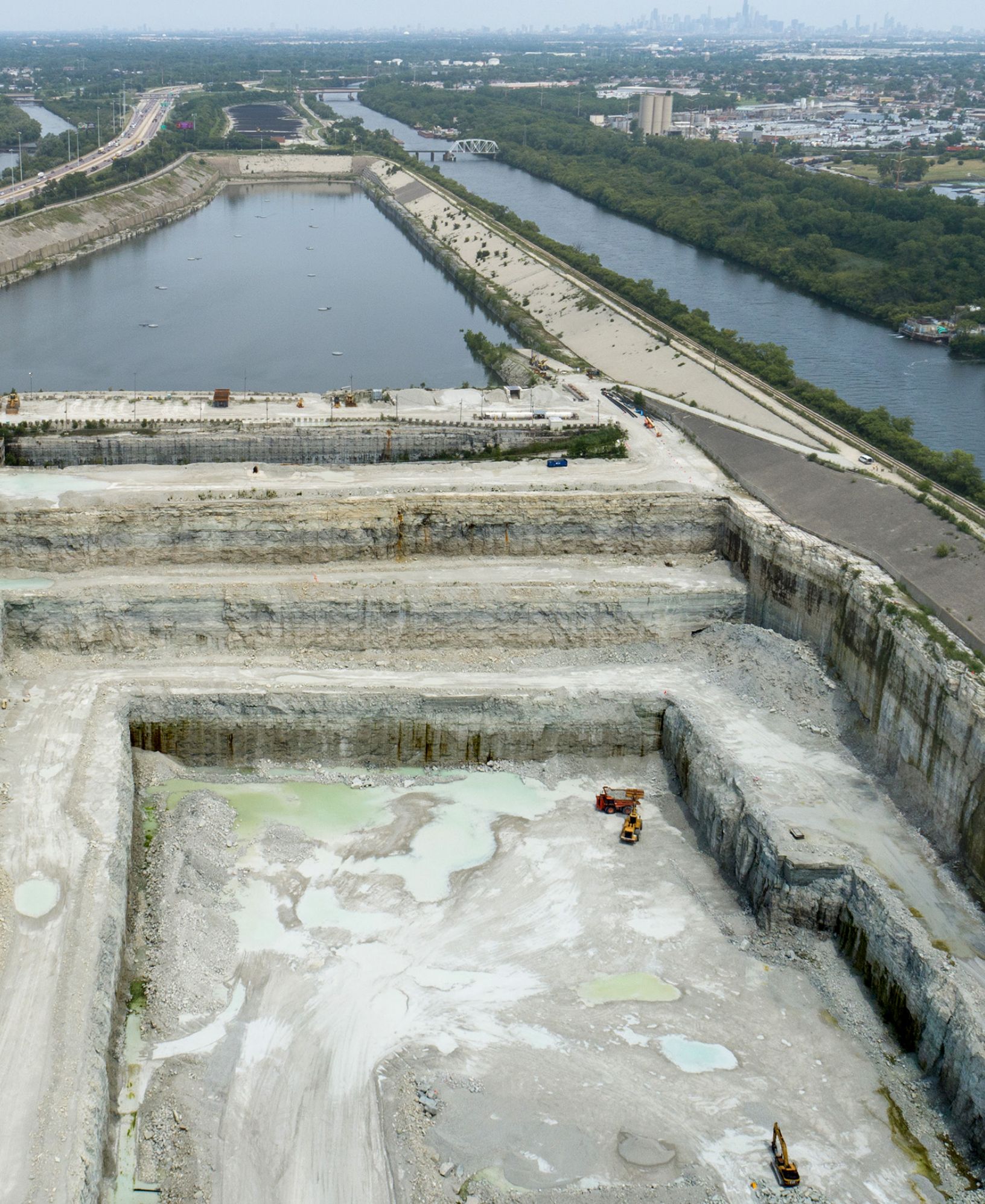
Phase 1 of the Tunnel and Reservoir Plan McCook Reservoir is in operation now as excavation is underway on Phase 2.
