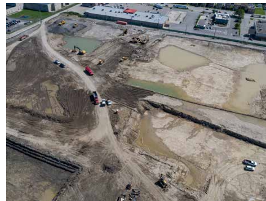
▼ Addison Creek Reservoir, 11-186-3F
