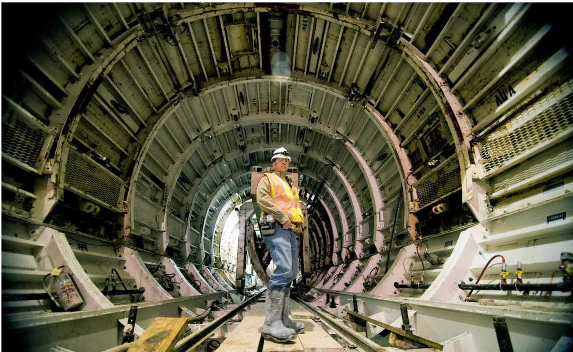
LEFT: A District engineer stands inside the formwork for installation of the concrete liner in the Des Plaines Inflow TARP Tunnel.
