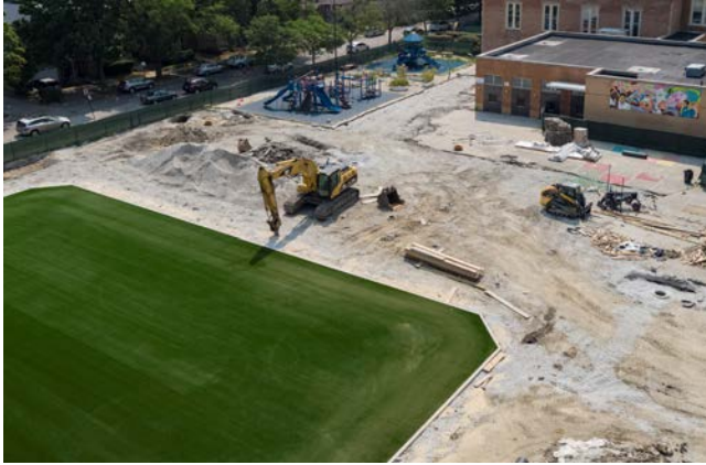
Construction on the Space to Grow schoolyard at Daniel Boone Elementary School.
