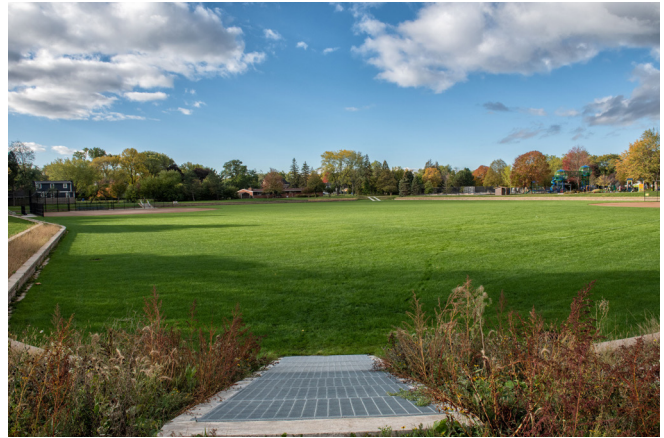
The first project completed at Burning Bush Trails Park included the construction of a detention basin.
