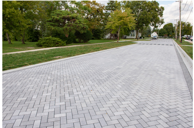
In Tinley Park, the MWRD contributed $200,000 to fund 16,500 square feet of permeable pavers and convert North Street into a green street. The project replaced the existing asphalt with green infrastructure that will provide more than 69,000 gallons of stormwater storage on site.
