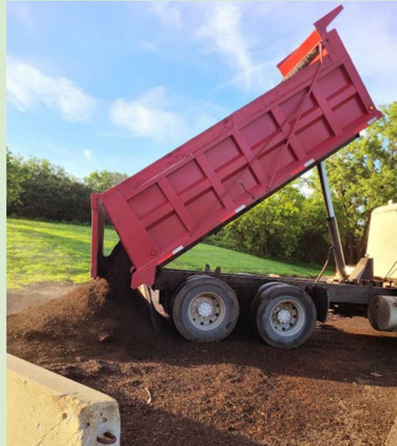
A dumptruck refills the empty site outside of the Stickney Water Reclamation Plant on June 16.
