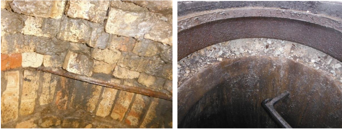
Figure 8.7. High-Priority Manhole Defects – Left: Deteriorating Brickwork; Right: Deteriorated Adjustment Ring
