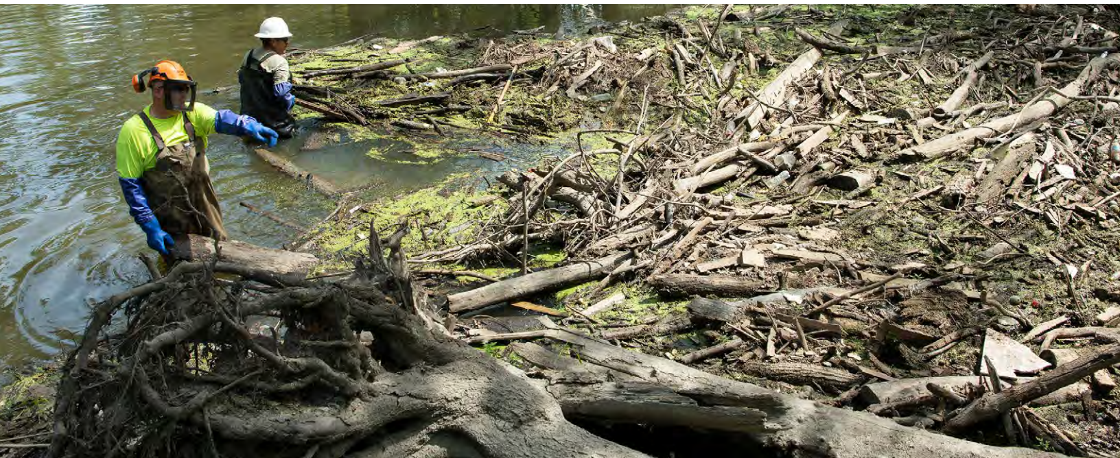
A crew removes a logjam in the North Branch of the Chicago River as part of the MWRD's Small Stream Maintenance Program.
